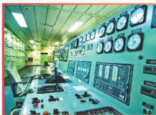
CUSTOM-TAILORED INTEGRATED ELECTRICAL, MECHANICAL, AND INSTRUMENTATION SOLUTIONS
